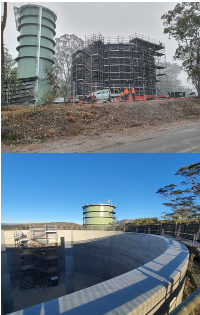
Figure 4: New steel and concrete reservoirs in Gloucester Water Supply System
