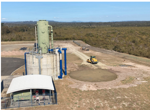
Figure 3: sub-base pavement and compaction completed for NABIAC Water Treatment Plant pre-treatment tank
