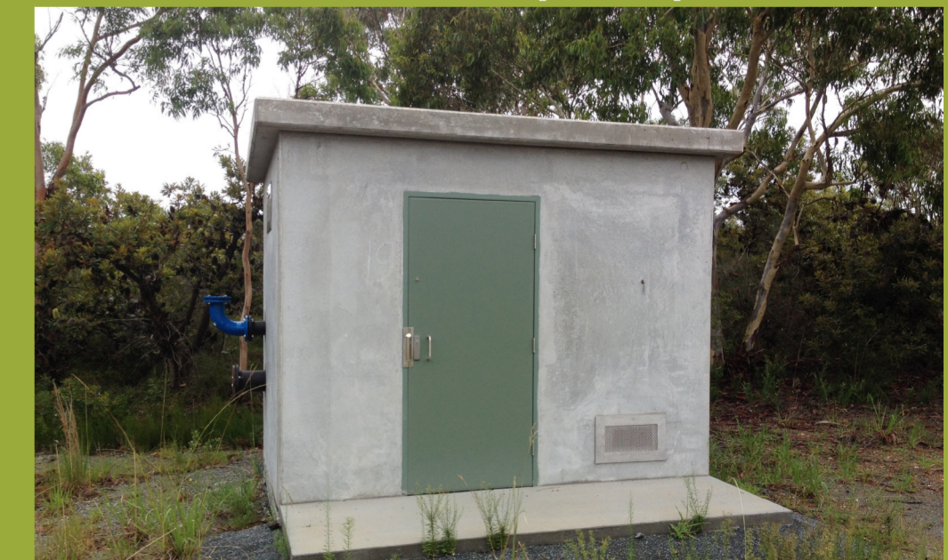
Production bore pump station
