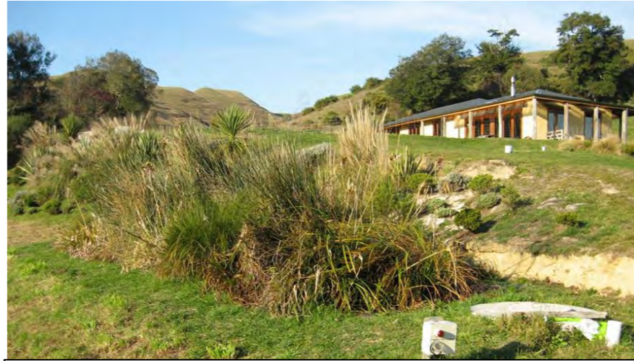
Reed bed – passively treats the wastewater using natural processes as it moves through vegetation.
