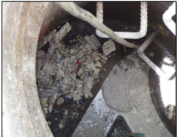
Figure 1. Sewer main, choked with fats (viewed down a manhole) caused by a food business operating with no grease arrestor.
