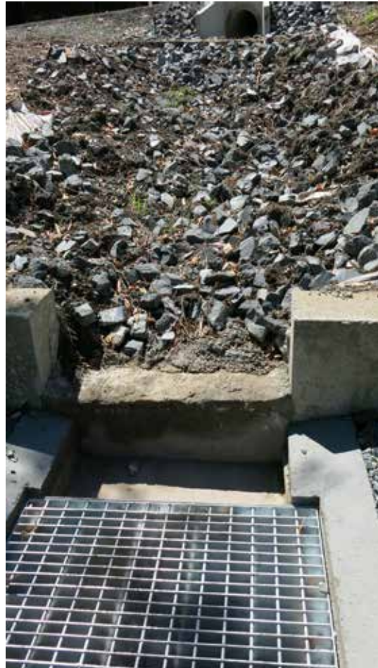
Figure 1.1.14 Rock lined drain and inlet pit at Tarbuck Bay
