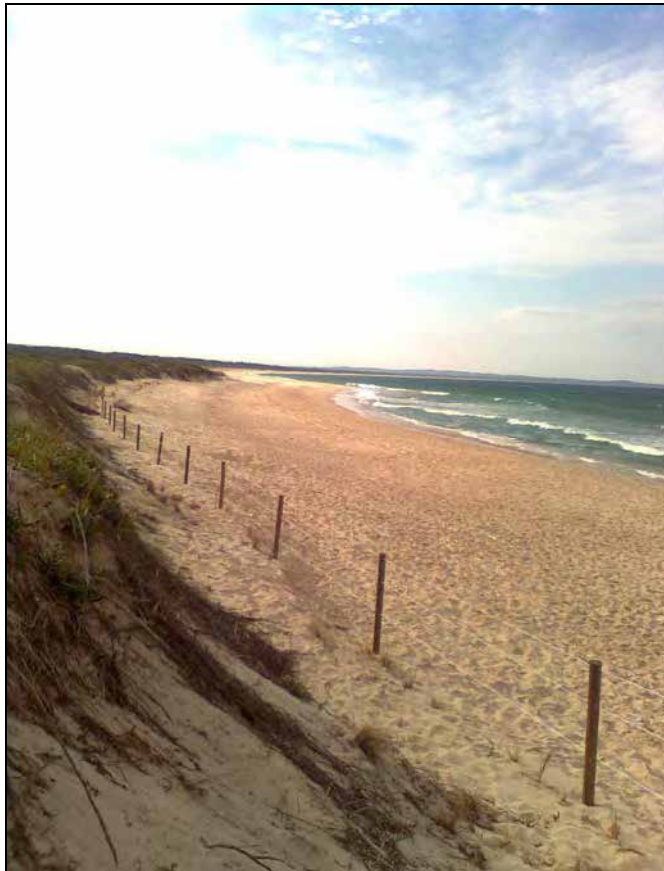
Figure 8.2 Evidence of eroded foredune at Tuncurry Beach
