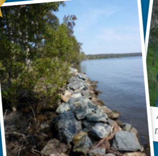
Stabilising 4.2km of the Wallamba River with rock protection, planting 8,000 native plants and conserving 8.6km of streambank
