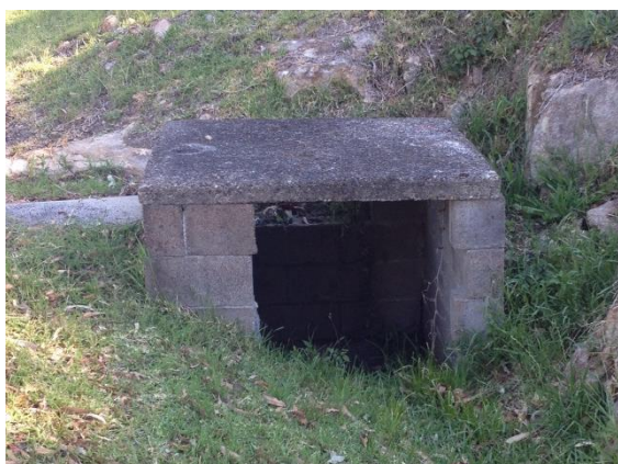
Figure 3-1 Example of hazardous pit inlet opening
