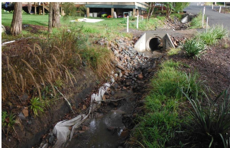
Figure 3-8 Lower Reach - undercutting of rock lining
