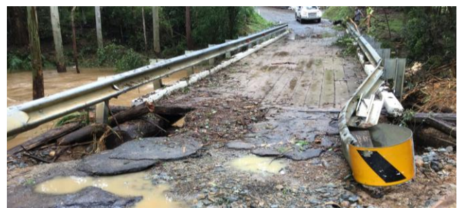
Starrs Creek Bridge damage on Waitui Road.
