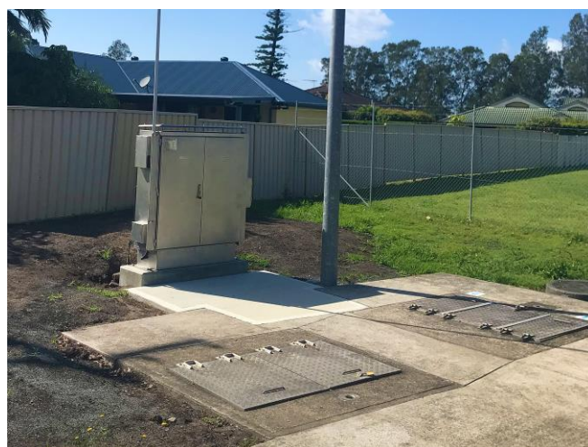
Solar power systems have recently been installed at our smaller water and sewer sites.
