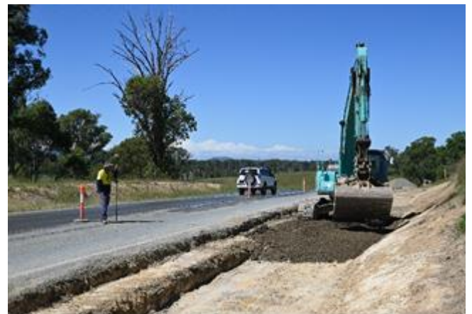
The Bucketts Way near Gloucester, as part of the $100 million Roads Program
