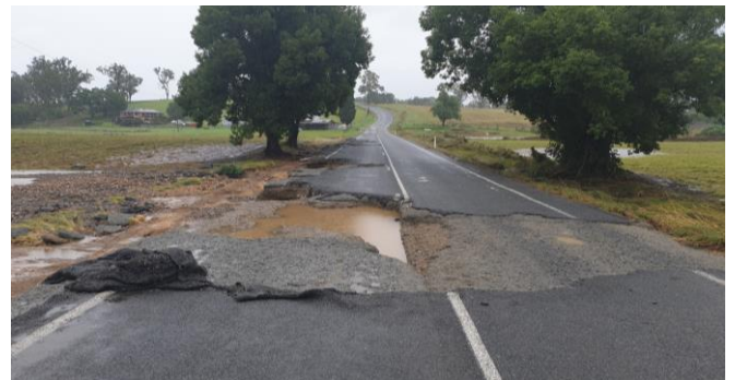
Gloucester Road compromised by flood damage.
