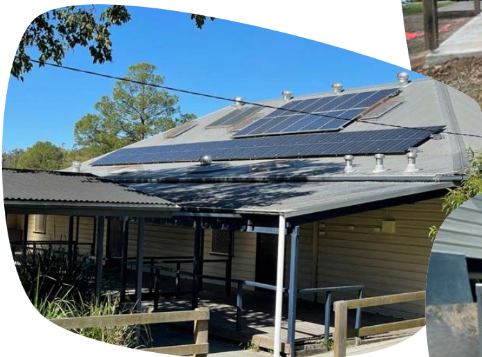
Above: Solar panels installed at Johns River Hall
