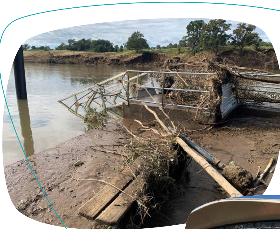
Damaged Wingham Brush Pontoon
