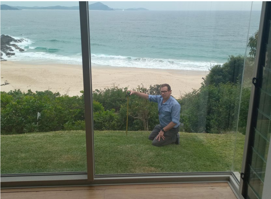
Figure 28 - View from the lower western section of the living area ground floor. The tape measure illustrates the height of the safety rail. (Source – Council staff inspection).
