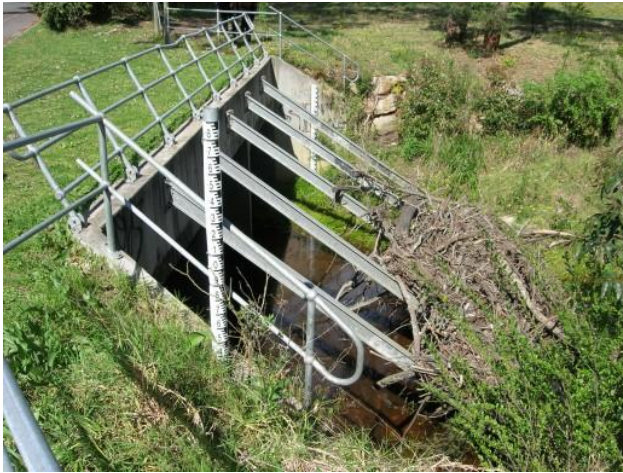
Photograph 11: Example of a rising deflection grate for prevention of culvert blockage
