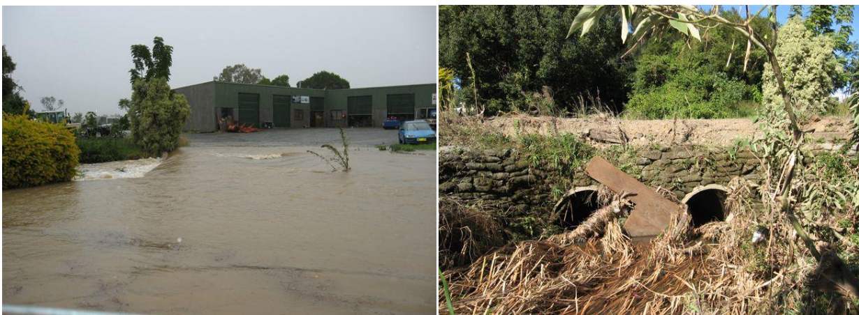
Photograph 7: “Industrial culverts” at Ferris Place overtopping in June 2007 (left), and afterwards partially blocked by debris (right). (Source: Bruce Weller)
