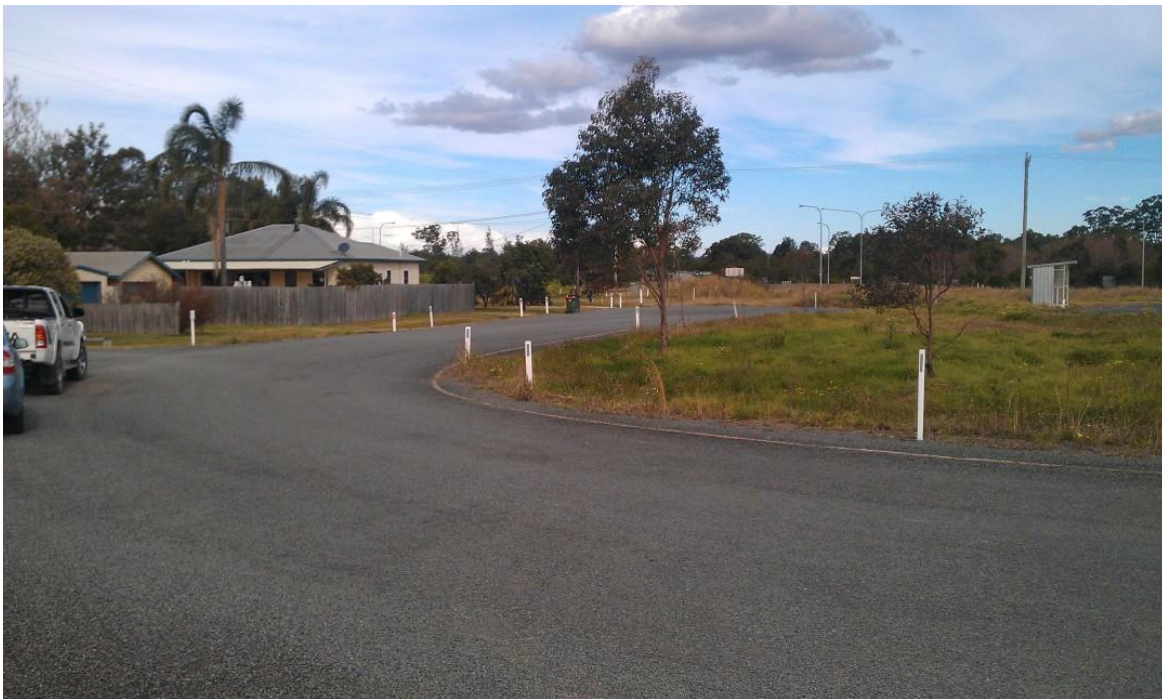
Photograph 17: Re-graded access to eastern end of Wallanbah Road, from Candoormakh Creek Road
