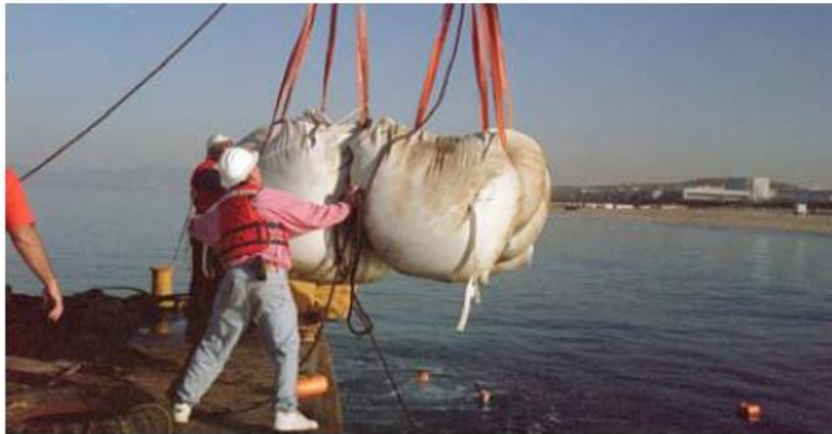
Figure 2.19: Placement of Smaller Geotextile Bags by Sling at Pratte's Reef (Borrero and Nelson, 2003; Jackson and Corbett, 2007)
