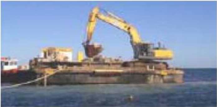
Figure 2.14: Placing Rock on the Cable Station Reef by Barge Mounted Excavator (Jackson and Corbett, 2007)
