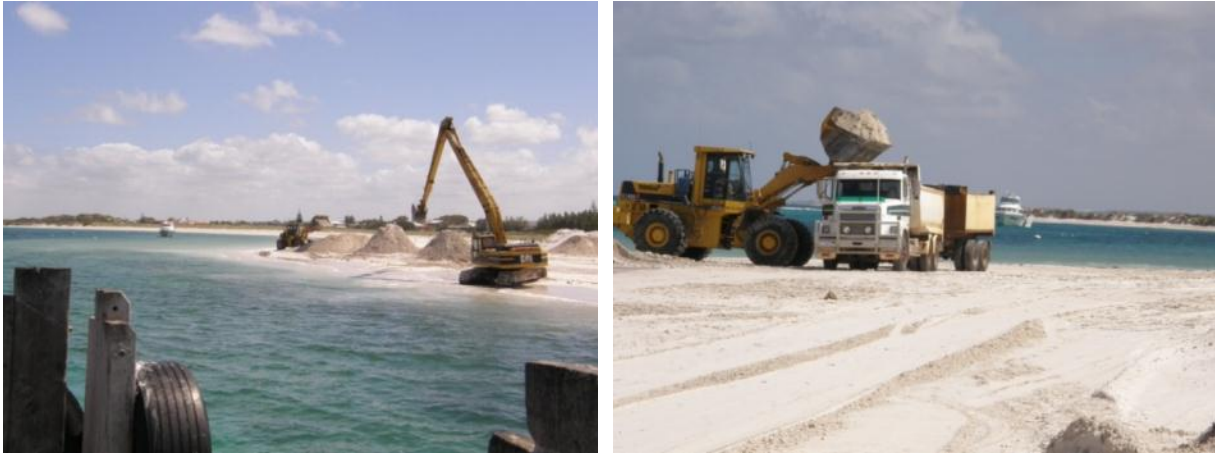
Figure 2-1 Land Based Plant methodology being used to excavate and haul material in Lancelin, Western Australia
