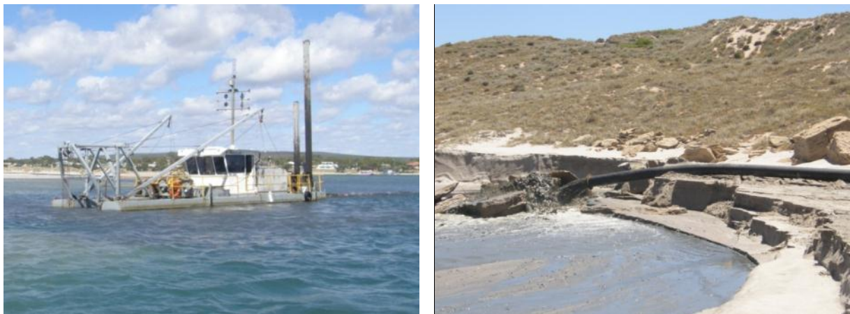
Figure 2-2 Floating Plant methodology being used to dredge material with a small CSD and being discharged directly onto the beach north of the Murchison River mouth, Kalbarri, Western Australia.
