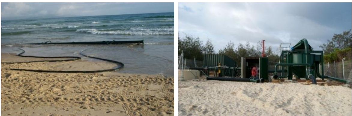
Figure 2-7 Sand shifter unit sourcing materials from the shore (left) with the associated onshore booster pumps and pipework (right) operating in Noosa , Queensland. (Source: Slurry Systems Marine)
