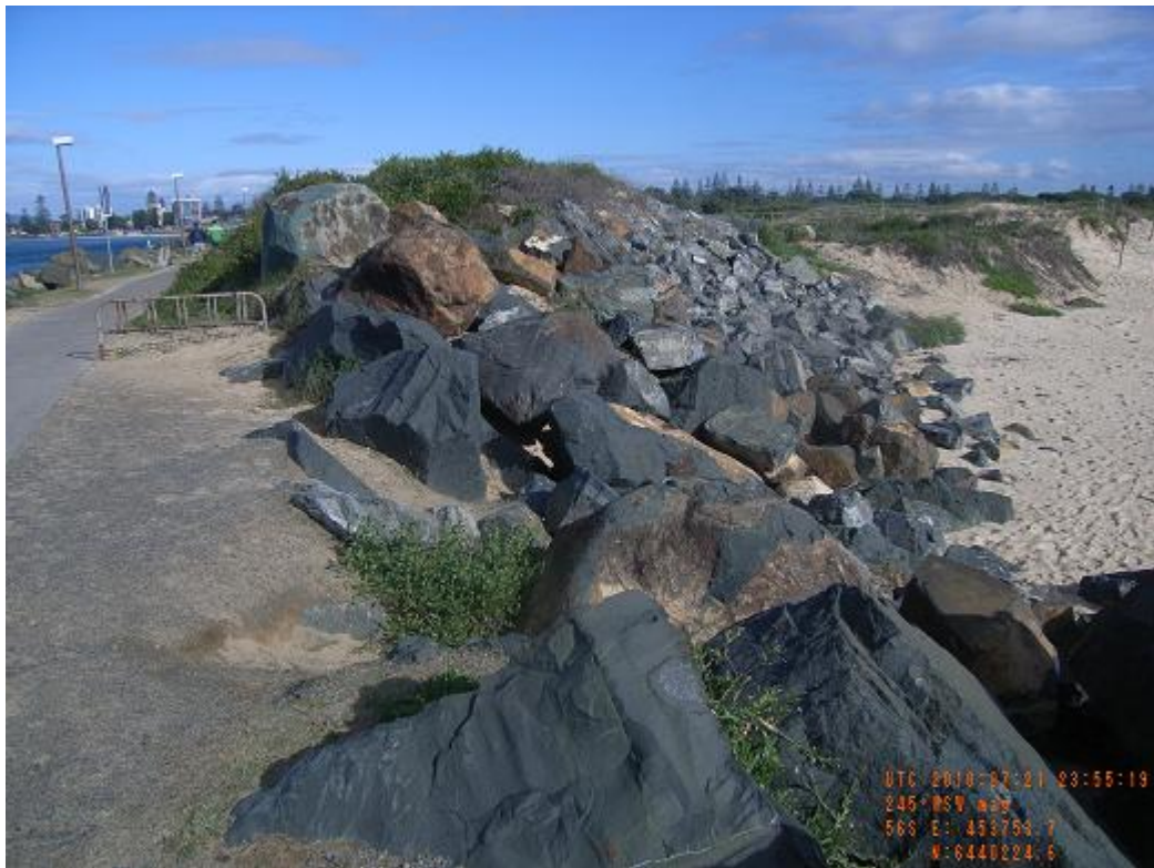
Figure 11: Failed seawall at the southern end of Nine Mile Beach and area of the seawall possibly subject to overtopping issues (July 2010)
