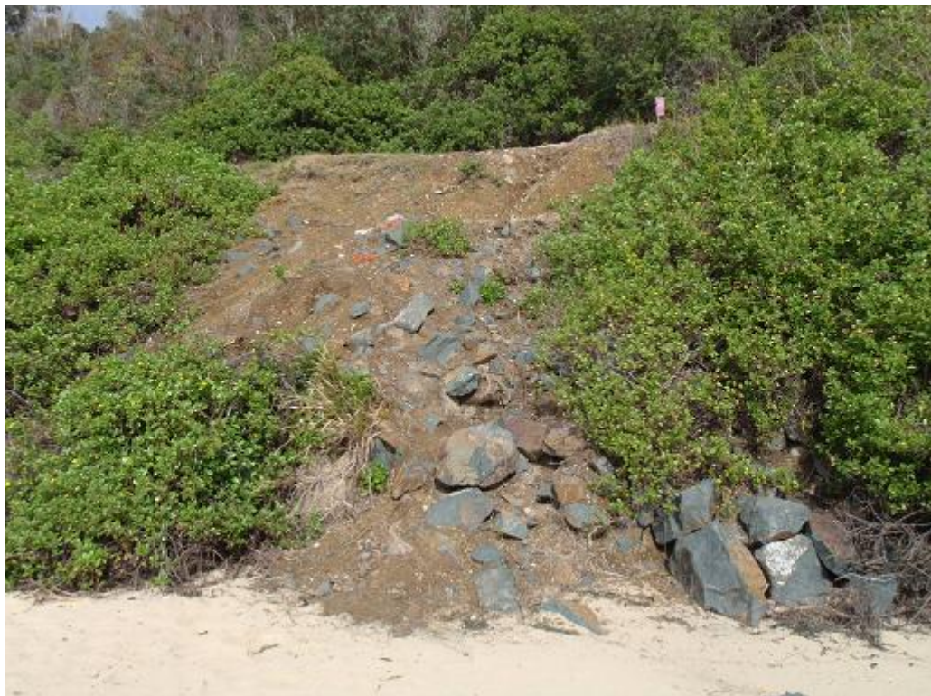
Figure 46: Landslip along Seal Rocks Road at Number One Beach (July 2010)
