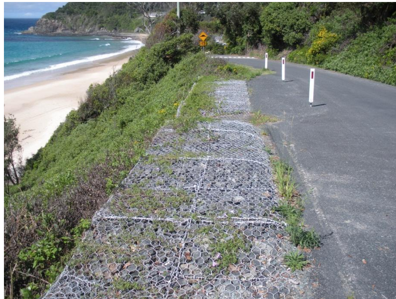
Photo 2: View of the gabion wall at the crest of the slope and alongside Kinka Road.
