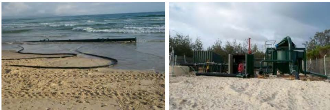
Figure 5 The Noosa trial Sand Shifter unit sourcing sand from the shore (left) and onshore booster pumps and pipework (right)
