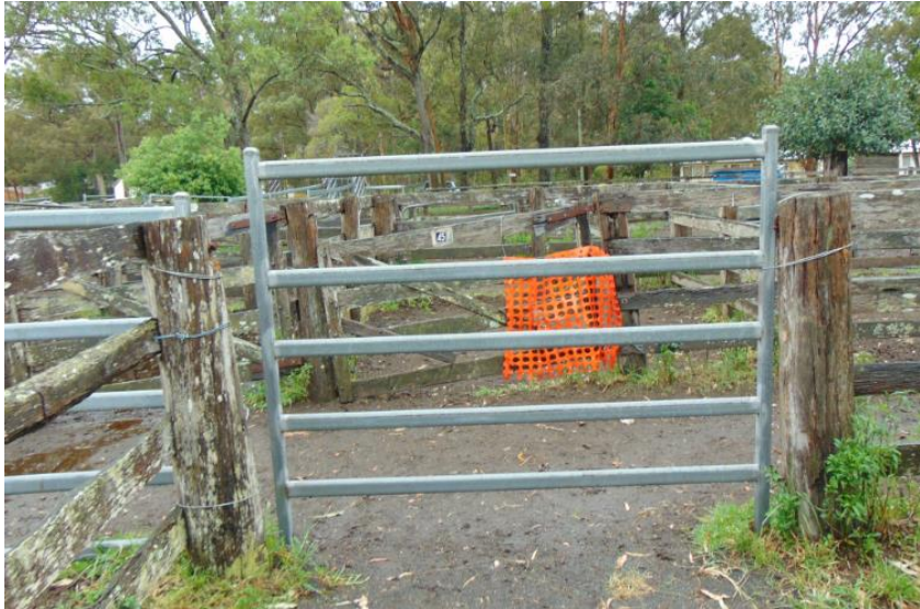
Figure 2 Yards repaired with wire and a mixture of panels
