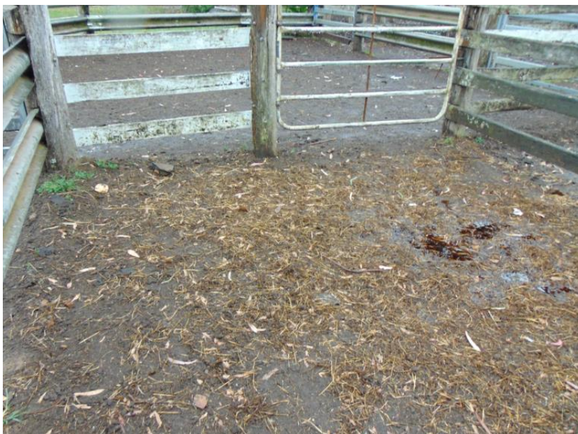
Figure 4 Dirt flooring with mud and effluent
