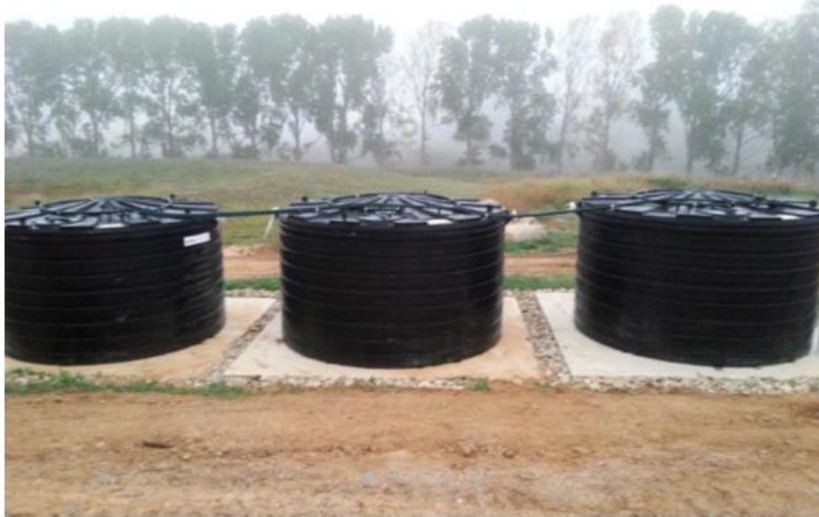
Figure 5 A Secondary effluent treatment system installed at the Braidwood Livestock Truck Wash (For Earth Pty Ltd)
